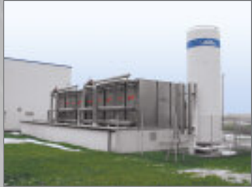
Industrial water cooling
