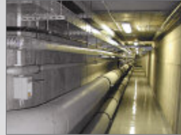
Underfloor supply pipes
