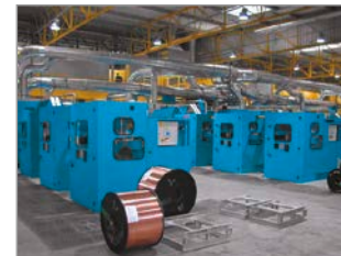
Exhaust air systems
