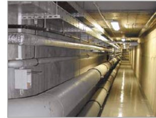
Underfloor supply pipes
