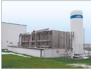
Industrial water cooling
